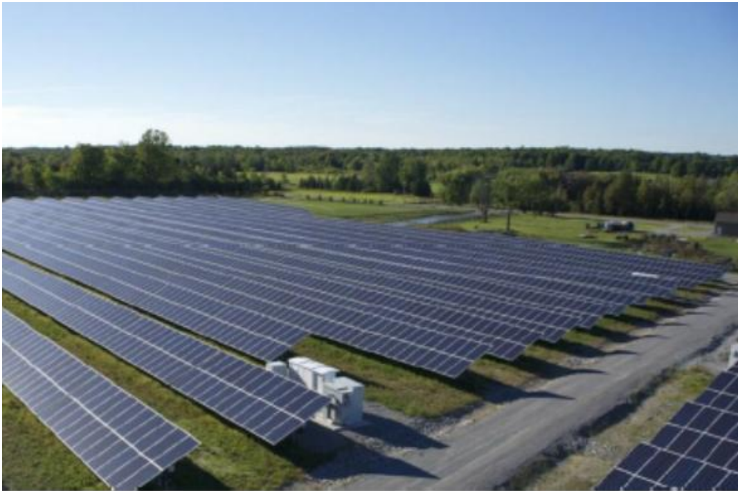
Image 4.2: Fixed South Facing PV Arrays
